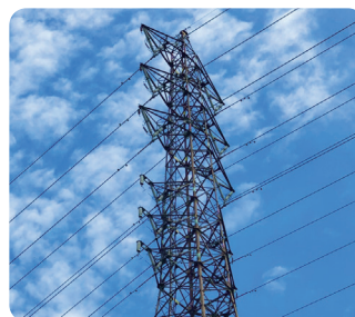
Transmission Towers/ Insulators
