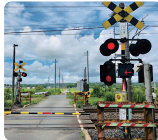
Sensors for Railways
