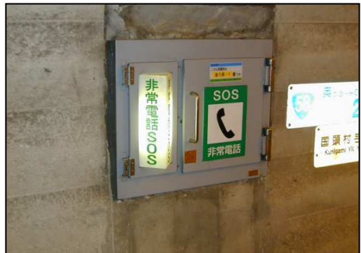
Telephone boxes in tunnels
